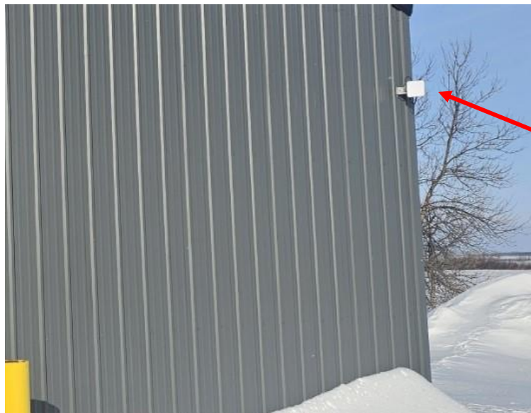
Wireless Camera Bridge mounted on outside of a new barn
